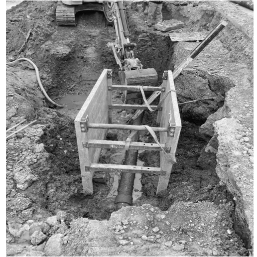
Mill Pond Water Main Break, 2022
